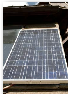
Photo Dan Fink - Typical solar electric panel (photovoltaic, or "PV"). (Photo 6)
