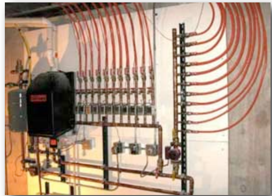
Photo Peak to Prairie Home Inspection Service - A typical solar hot water system control center. (Photo 9)
