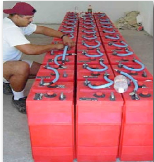
Photo Northern Arizona Wind and Sun A large battery bank, used to power a home during a utility grid blackout. (Photo 2)
